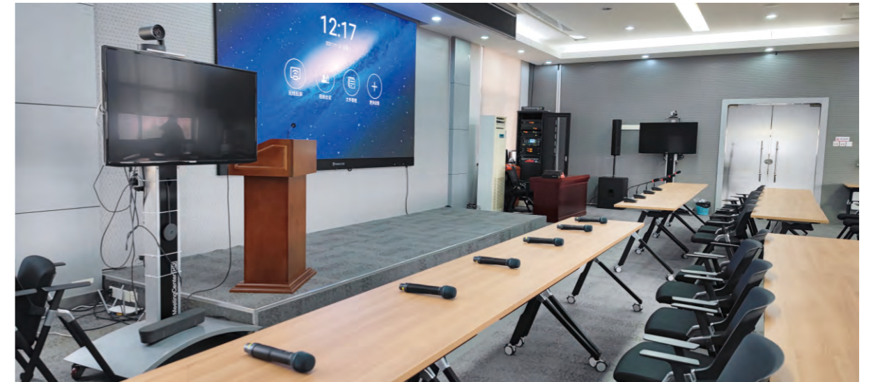
WAM-432+UR-260D | WAM-432 automatic intelligent wireless mixing system was installed in Shandong Province for staff training
